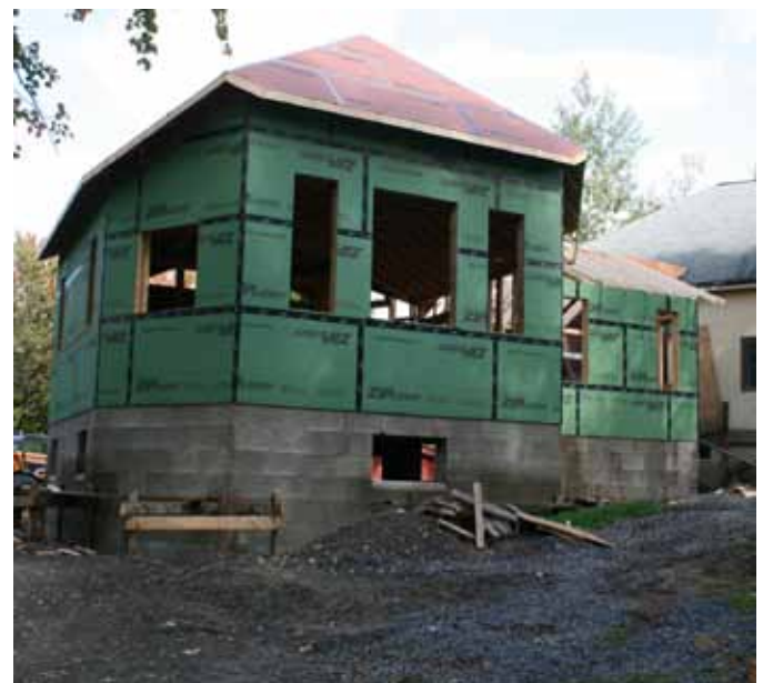
By the end of September the outer shell was nearly finished and we could experience the building in its final size and proportion. It's a beautiful structure and we aim to be using it by February.
